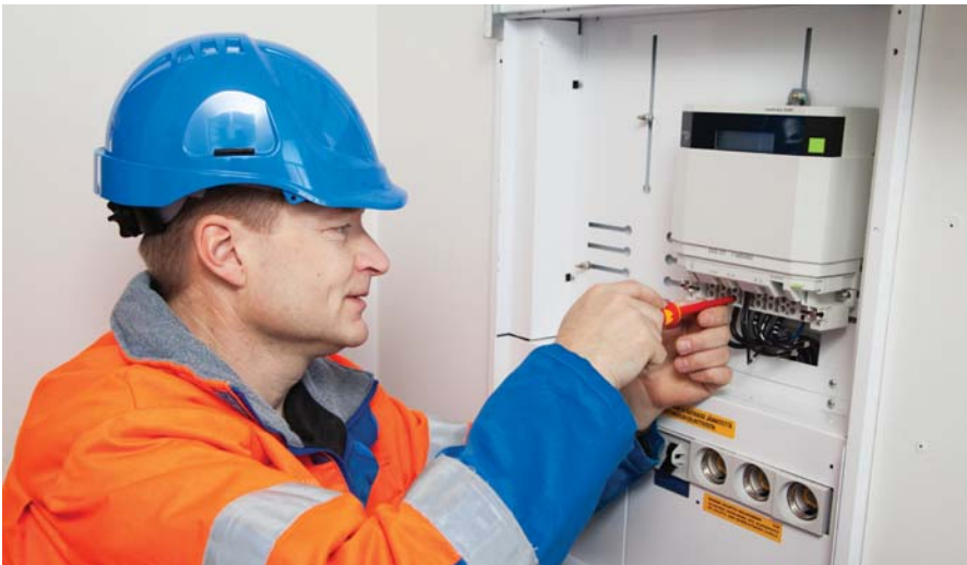
The mass-roll out of smart meters and implementation of smart metering is carried out in phases by geographical areas. This enables the utility to benefit from smart metering already in the early phases of the project. Smart meters are installed by Suur-Savon Sähkötyö Oy.
